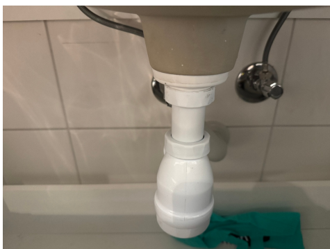
Røropplegg under servant.
