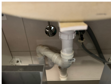
Røropplegg under servant.
