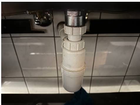
Røropplegg under servant.
