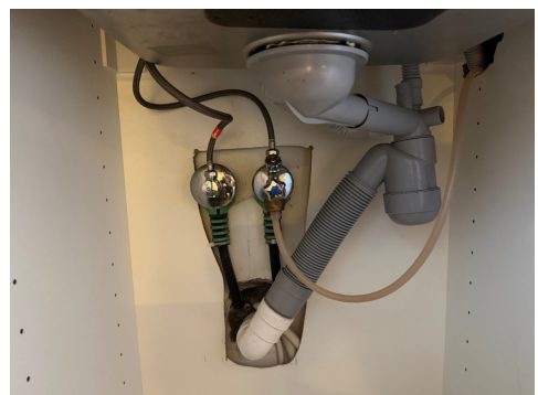
Røropplegg under vask.
