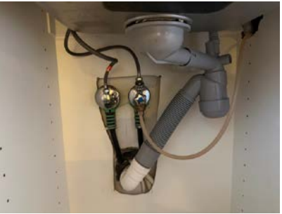
Røropplegg under vask.
