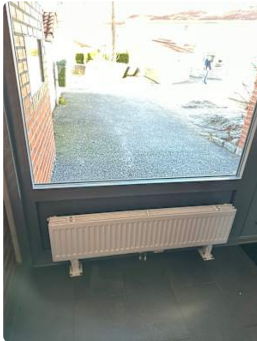
Radiator i fellesareal
