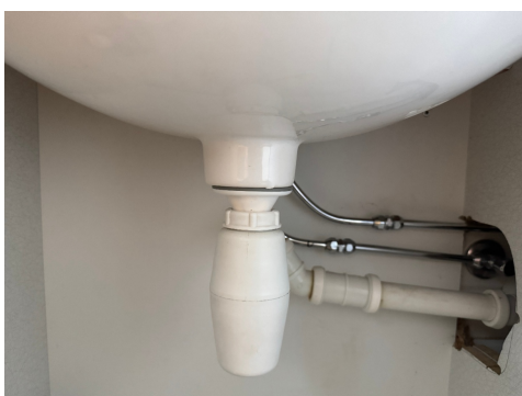
Rørplegg under servant.
