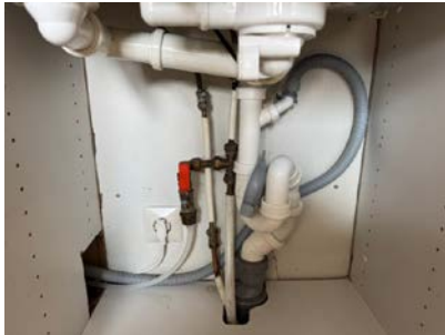
Røropplegg under vask.
