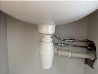
Rørapplegg under servant.
