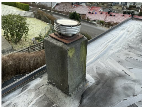
Noe slitt inntekking.
