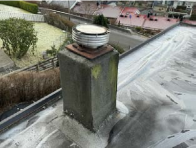
Noe slitt inntekking.
