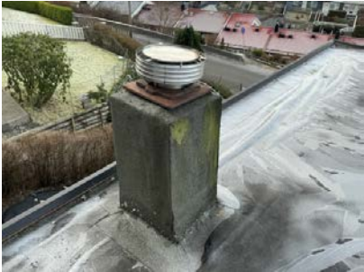
Noe slitt inntekking.
