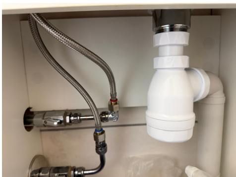
Røropplegg under servant.
