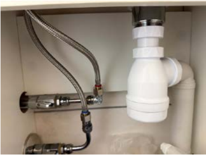
Røropplegg under servant.
