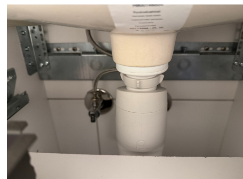
Rørpropp under servant.
