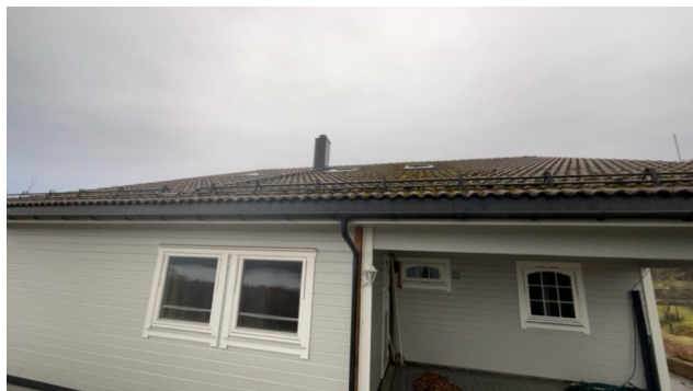
Takstein, noe mose
