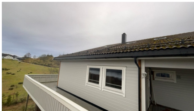
Takstein, noe mose
