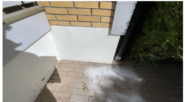
Stedvis riss i murpuss/maling.
