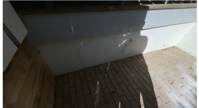
Stedvis riss i murpuss/maling.
