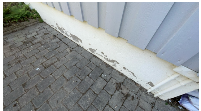
Stedvis riss i murpuss/maling.
