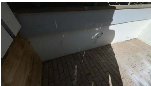
Stedvis riss i murpuss/maling.
