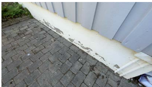
Stedvis riss i murpuss/maling.
