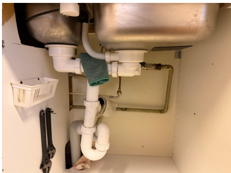
Røropplegg under vask.
