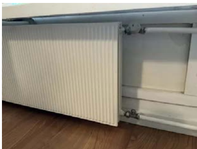
Radiator i stue.
