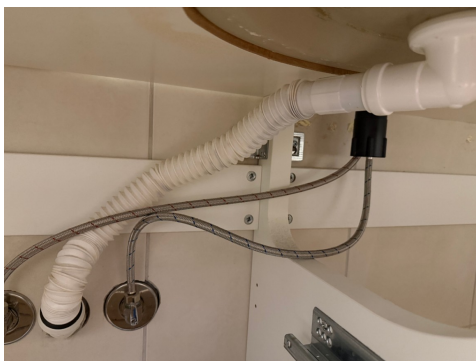
Røropplegg under servant.
