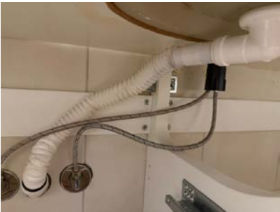
Rørapplegg under servant.
