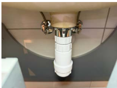
Røropplegg under servant.
