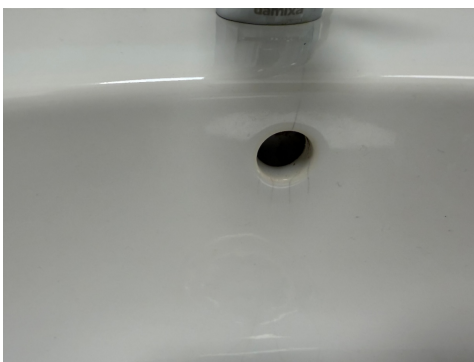
Riss/krakelering i servant.
