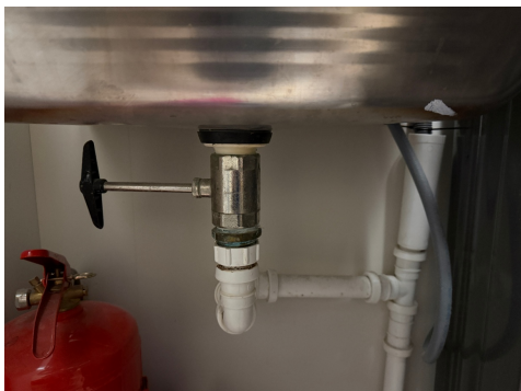
Røropplegg under vask.
