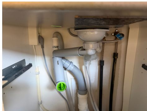
Røropplegg under vask.
