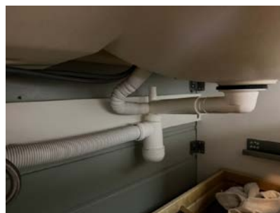
Røropplegg under servant.
