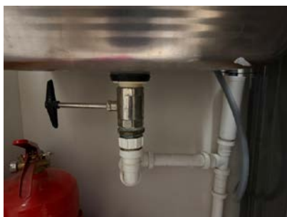
Røropplegg under vask.
