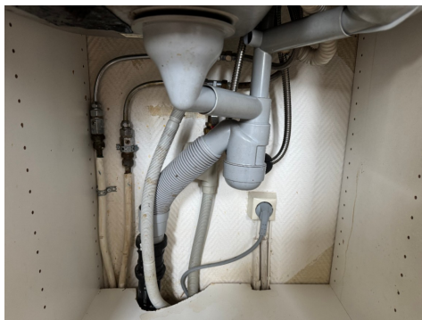
Røropplegg under vask.
