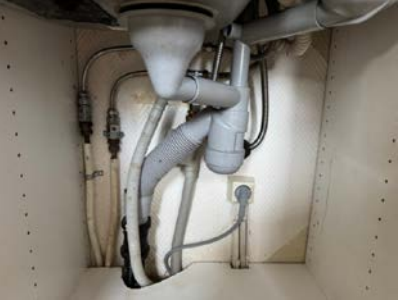
Røropplegg under vask.
