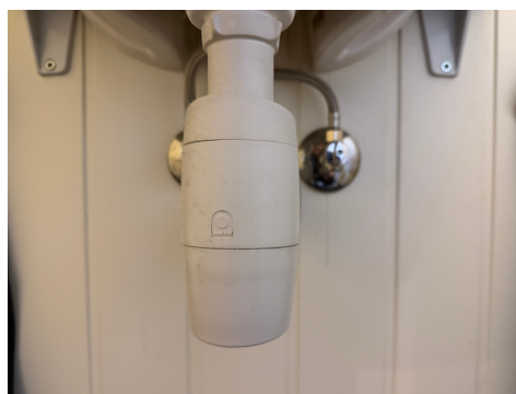
Rørproppleg under servant.
