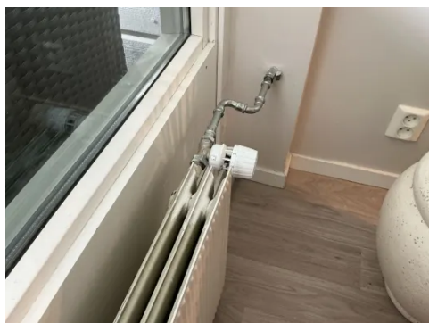
Radiator i stue.
