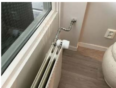
Radiator i stue.
