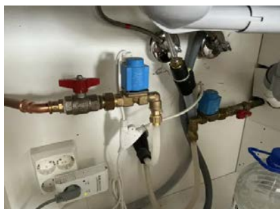
Stoppekran under kjøkkenvask.
