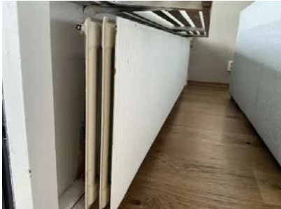
Radiator i stue.
