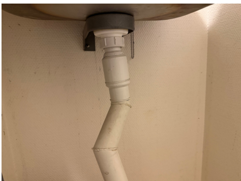
Røropplegg under vask.
