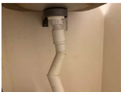
Røropplegg under vask.
