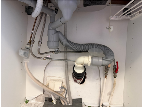
Røropplegg under vask.
