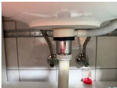
Røropplegg under servant.
