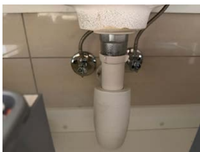
Røropplegg under servant.
