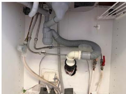
Røropplegg under vask.
