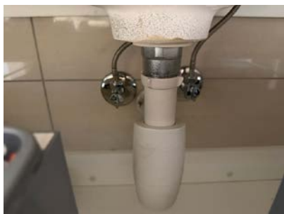
Røropplegg under servant.
