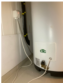
Bereder i bod under trapp, fast EL-tilkopling
