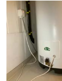
Bereder i bod under trapp, fast EL-tilkopling
