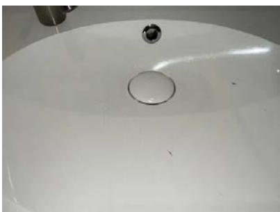
Krakelering i servant.
