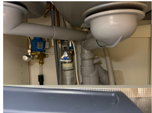
Rørpropplegg under vask.
