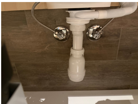
Røropplegg under servant.
