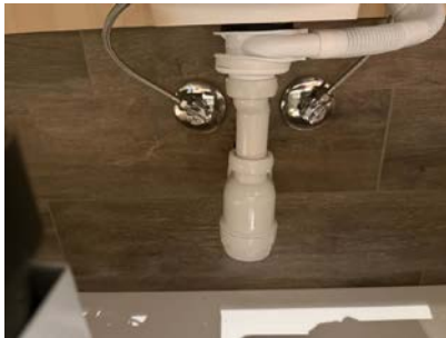
Røropplegg under servant.
