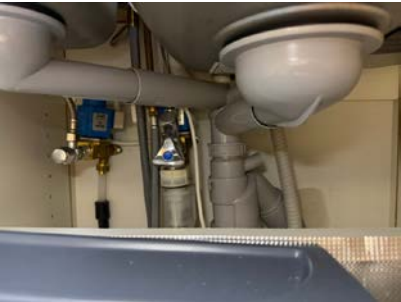
Røropplegg under vask.
