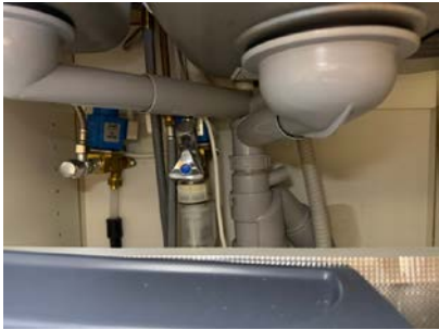
Røropplegg under vask.
