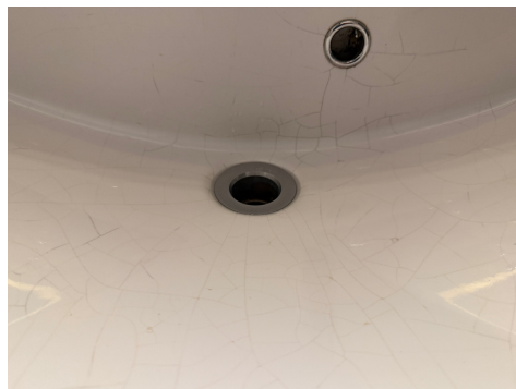
Riss/krakelering i servant.
