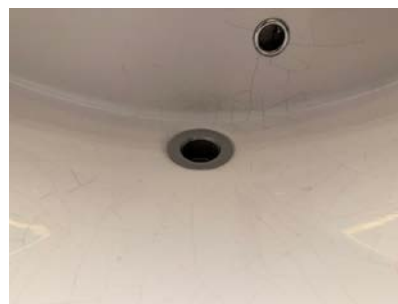
Riss/krakelering i servant.
