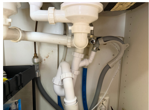
Røropplegg under vask.
