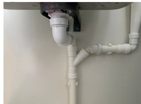
Røropplegg under vask.
