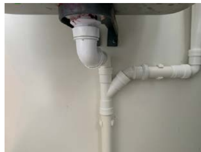
Røropplegg under vask.
